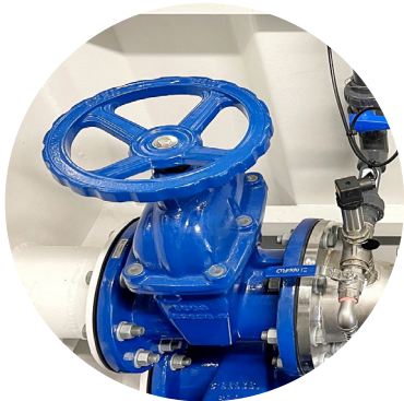
External mixer aerator pump combination
