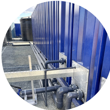
Interconnection provisional flanges for rapid set-up
