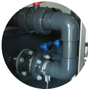
Grey UPVC sch 80 pipe work, valves & fittings
