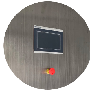
Fully automated control with Allen Bradley HMI & PLC
